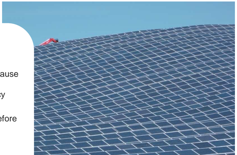
18.2 MWp installation in Les Mées in South of France.
