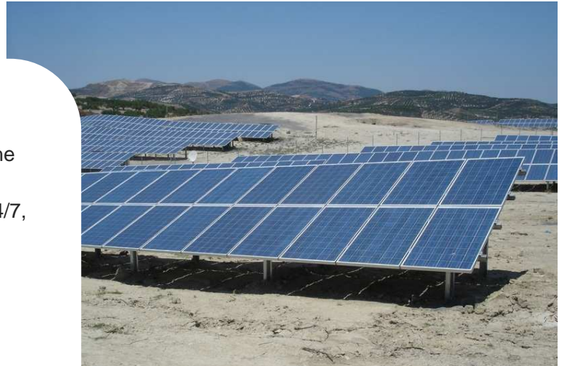
1 MWp ground mounted installation in Greece.
